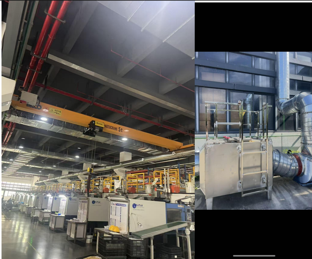
注塑车间废气收集、活性炭吸附
